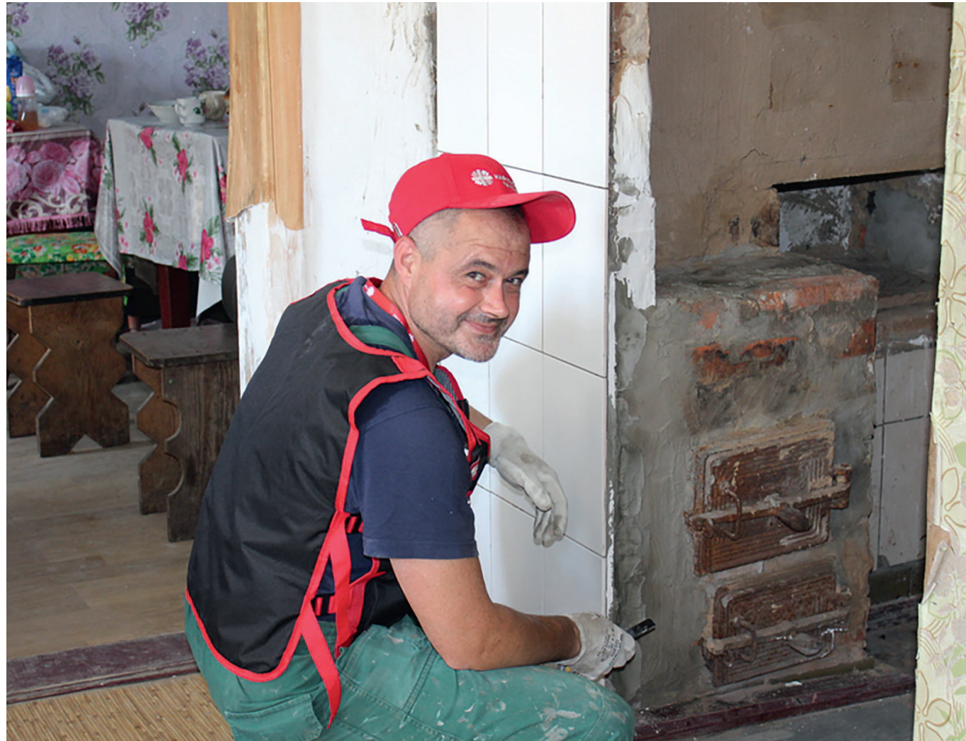
Worker of a construction team restoring a damaged building. Photo by Tetiana Kalinichenko. Sloboda village, Chernihiv region. Summer of 2022
